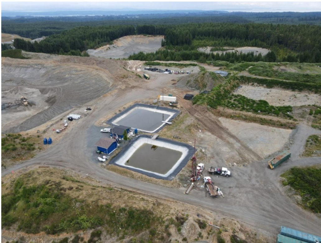
Photo 3-1: Leachate Treatment Ponds – Photo taken June 2025
