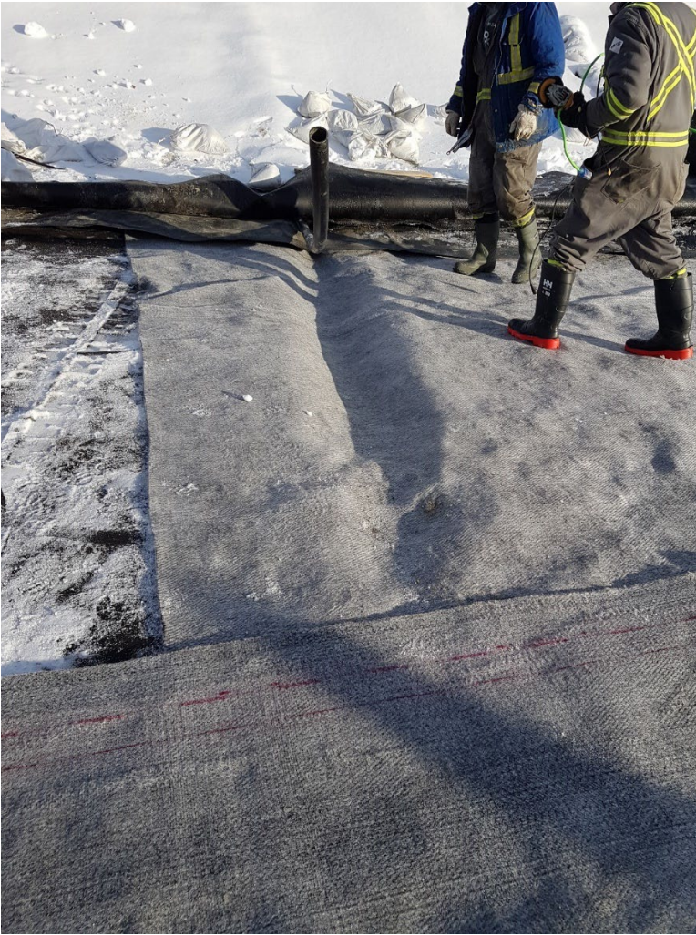
Photo 19 50 mm Leak Detection Riser Pipe
