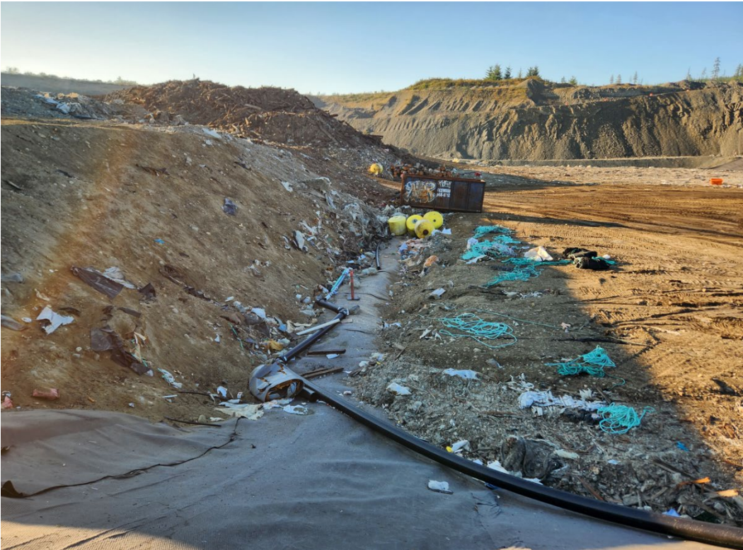
Photo 27 Pipe directing leachate to Cell 1 East (September 22, 2023)
