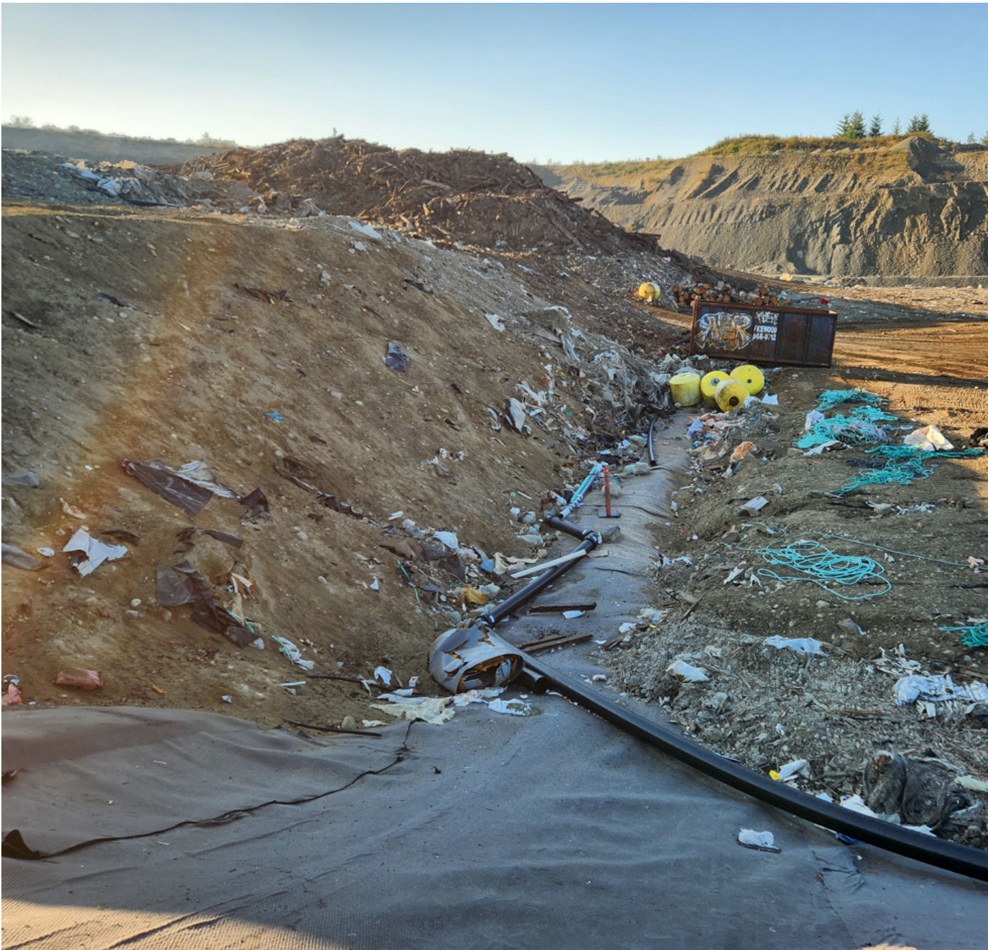
Pipe directing leachate to Cell 1 East
