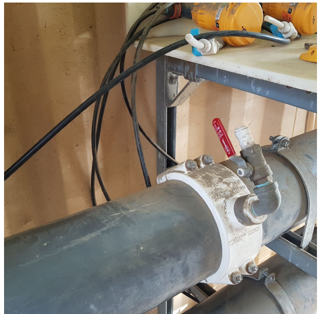
Photo 8 Typical chemical injection port
