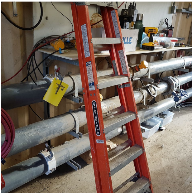
Photo 7 Leachate and effluent lines inside treatment container
