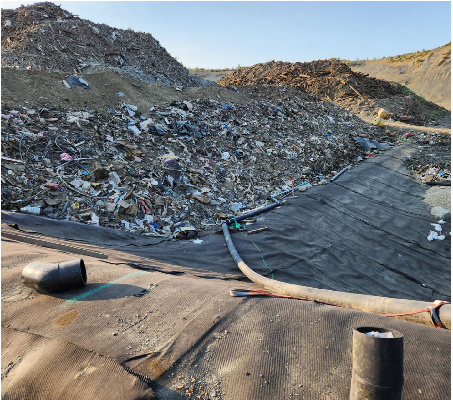
HDPE pipe connected to leachate collection pipe in Cell 1 East
