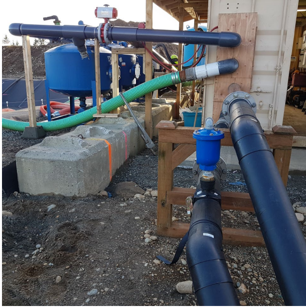
Photo 5 Leachate inlet / effluent out lines
